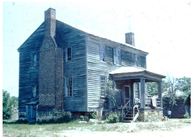
Dromgoole House before it was wrapped in Tyvex—a white weather resistant plastic to prevent further deterioration.
