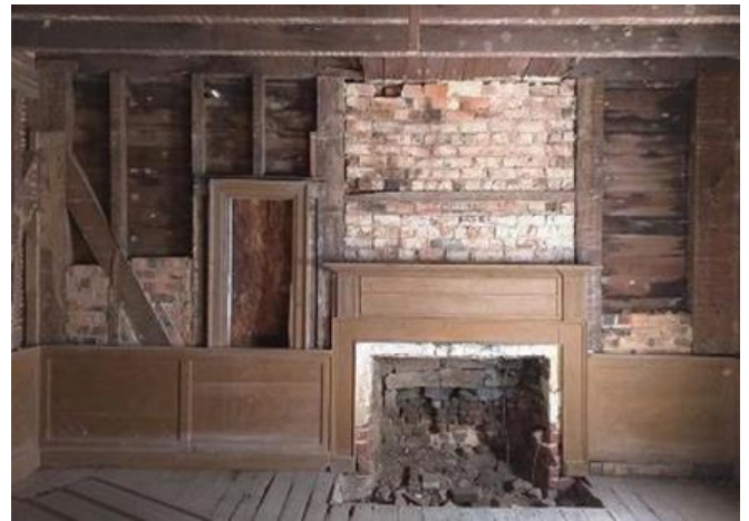
Interior of the Dromgoole House showing architectural features such as the mantel and brick "nogging" in the walls.
