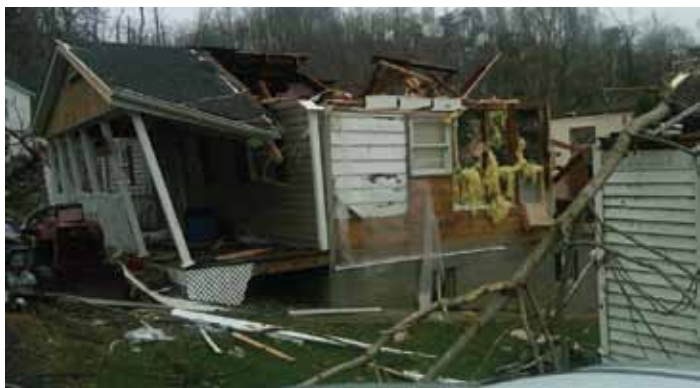
New houses to replace tornado-damaged homes such as this one in Pulaski are being built by disaster response volunteers. (VDEM photo)
